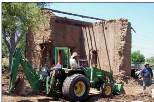
Emergency stabilization work at the steam pump building summer 2007. Historic adobes were saved for future restoration.
